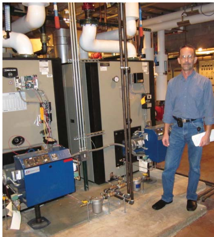
Chief of Maintenance and Security Al Dallasta with the new dual-fuel boilers.
